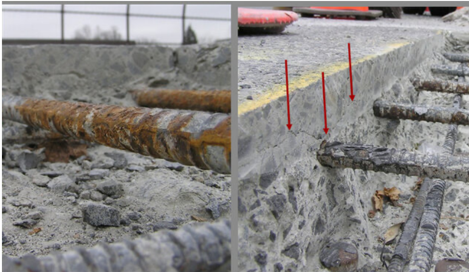
Figure 2: Typical concrete bridge deck deterioration and damage: rebar corrosion (left), delamination (middle) [5]
